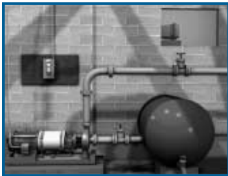
Software embedded in the controller micro-processor becomes the "brains" of a pumping system.
